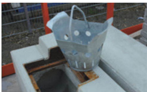
Installed sump unit
